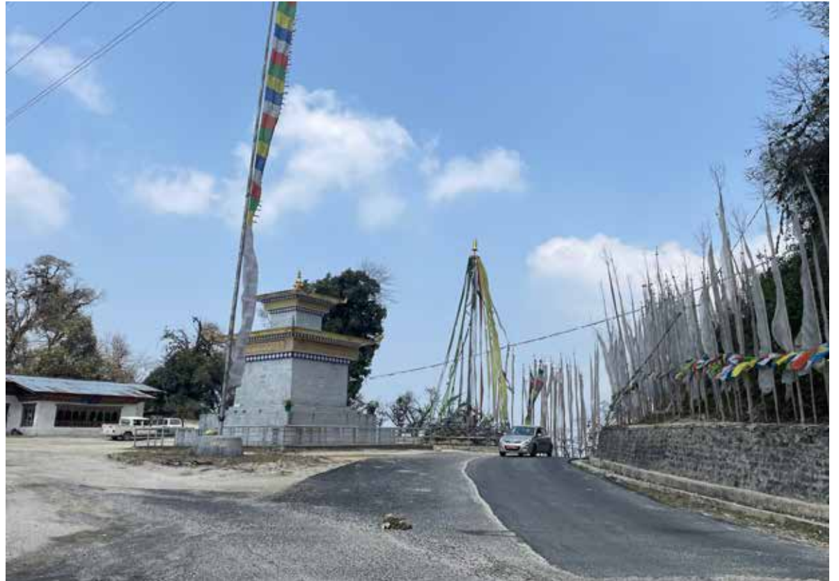
► The widening and blacktopping of the Korila-Ngatshang road on Mongar-Trashigang highway that started in March 2019 have been completed. The road is expected to be handed over to authorities soon. ► Pg 13
